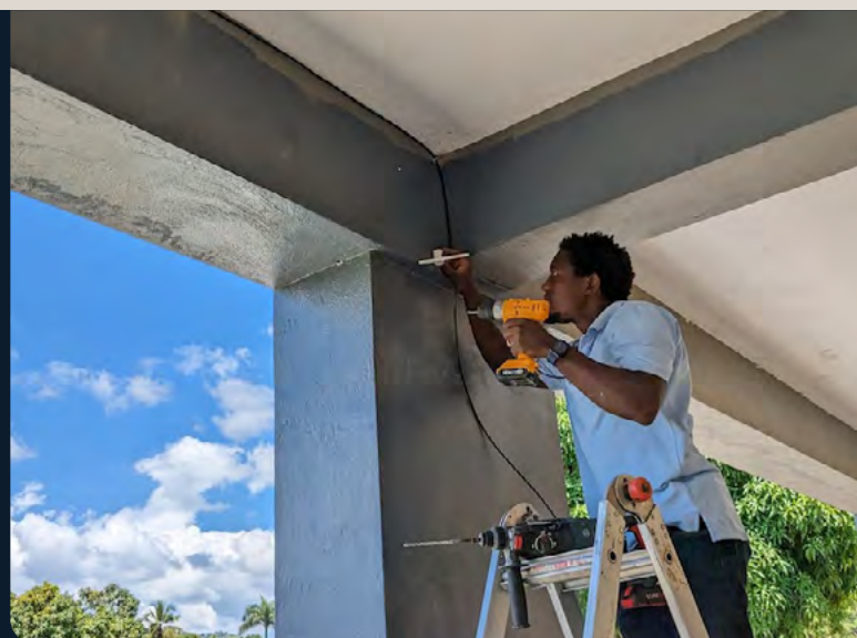
Haiti Chapter installs networking equipment to connect communities across the island. © Internet Society Haiti Chapter
