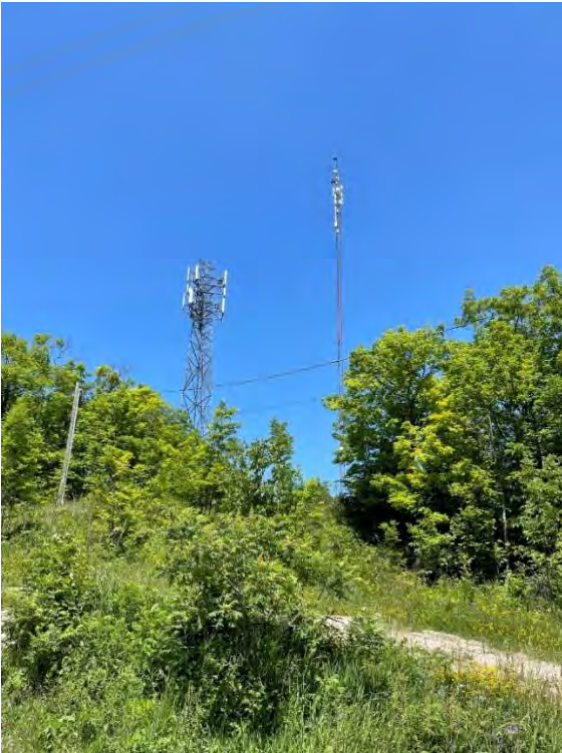
Microwave radio-based tower serving Nawash
